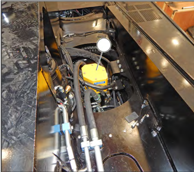
Figure 307: Check and cleaning of the transmitter rings of the rotating electric collector
