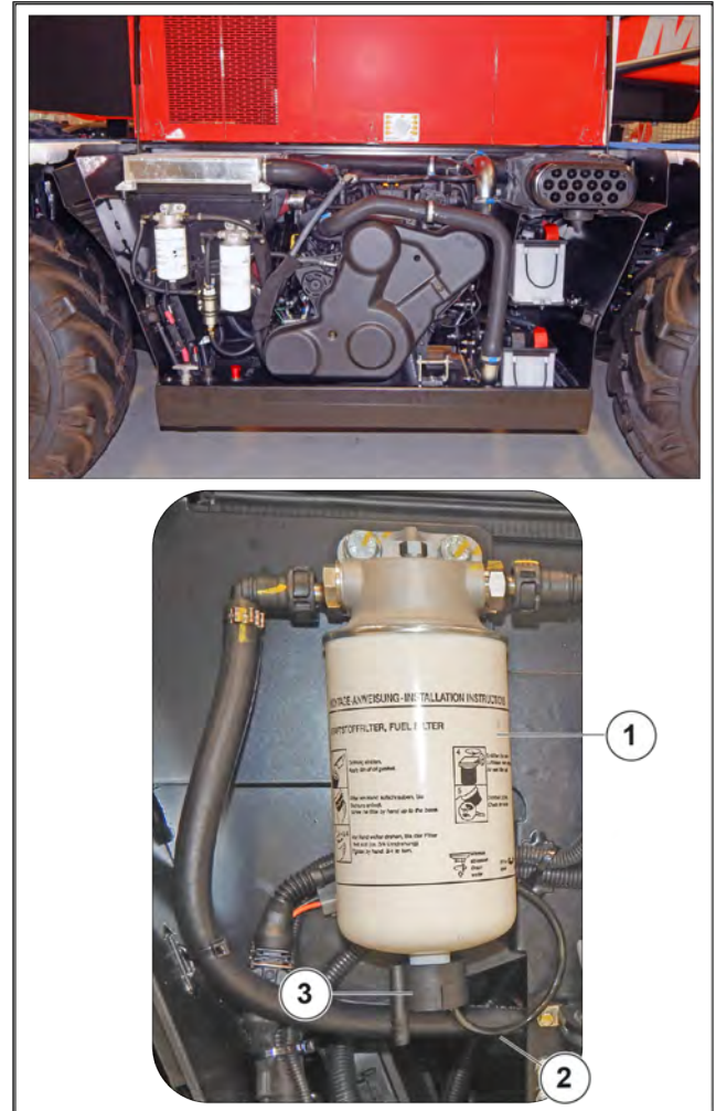
Figure 242: Fuel pre-filter check
