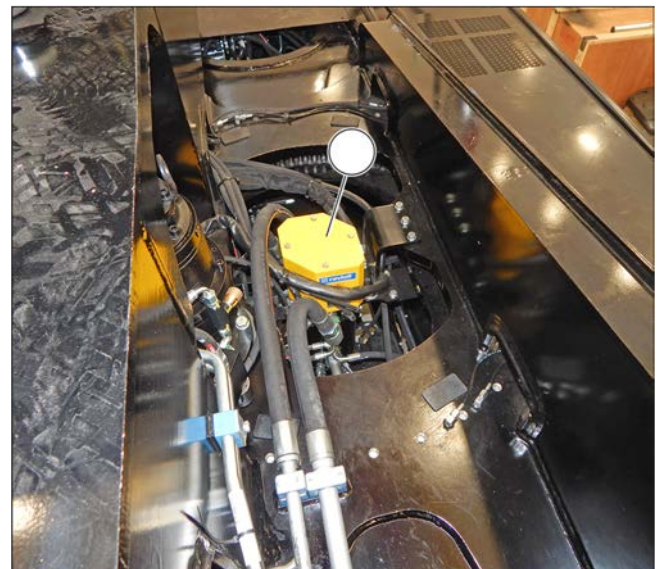
Figure 224: Check and cleaning of the transmitter rings of the rotating electric collector
