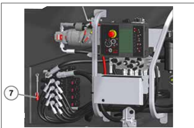
Figure 50: Location of the emergency controls 2
