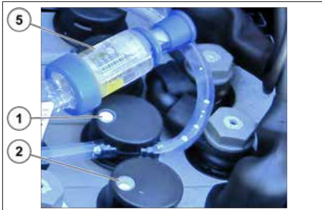
Figure 26: Manual centralized filling of high-voltage batteries 1
